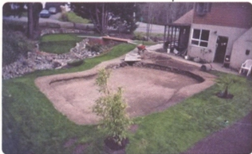
Rob Crompton began construction of his USGA-style backyard golf hole by digging out the green cavity with a pick and shovel.
